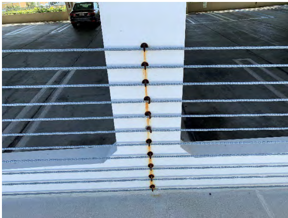
Photograph 5: Rusting guard cable eyes
