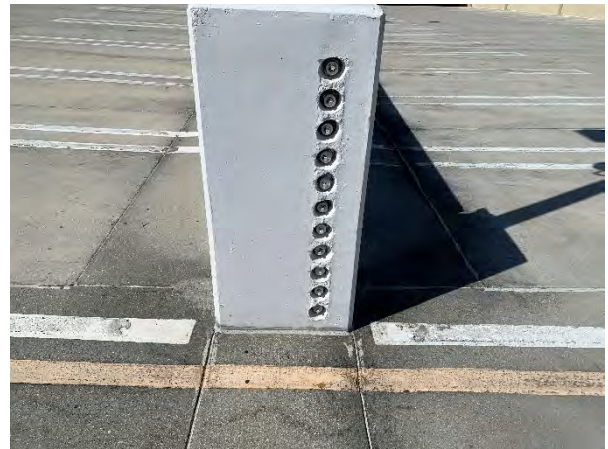
Photo 6: Exposed post tension cable ends
