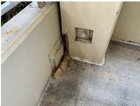
Photograph 7: Spalling of rebar and failed cant head
