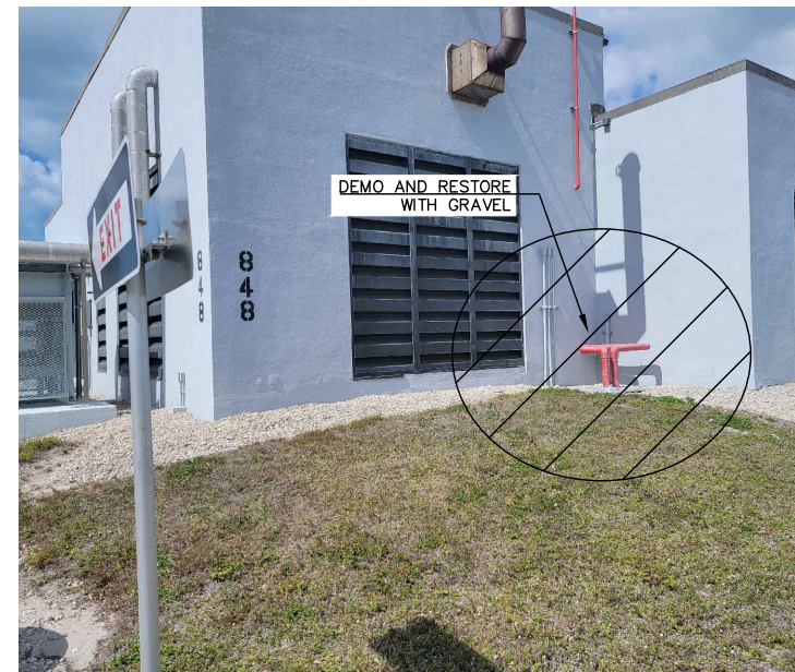
EX. DIESEL WELL GEN #1
