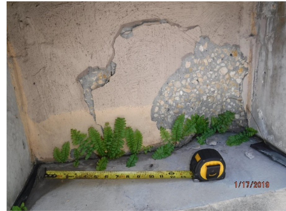
PHOTO 2 - VEGETATION AT END BENT 1 AND SPALL AT DIAPHRAGM BETWEEN SLAB UNIT 1-12 AND THE COSMETIC FASCIA BEAM.
