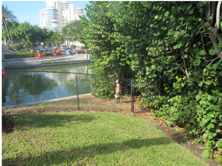
PHOTO 13 - REPLACE FENCE AND GATE AT END LEFT QUADRANT.
