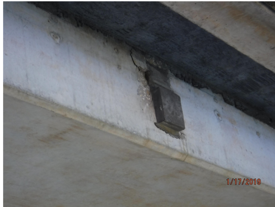
PHOTO 5 - SPALL AT NORTH FACE OF SLAB UNIT 4-1 AT POST-TENSION DUCT
