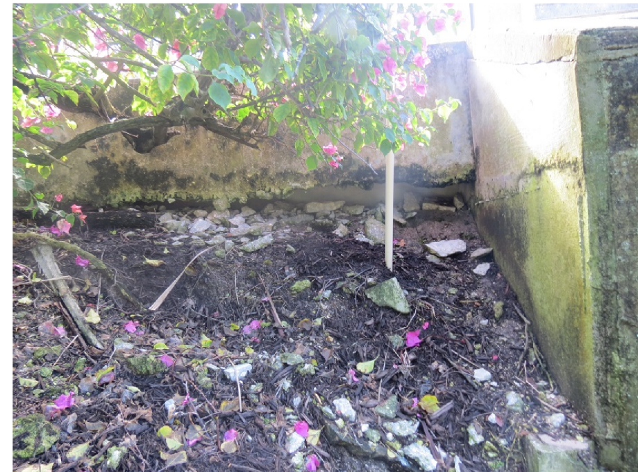
PHOTO 8 - UNDERMINING AT SIDEWALK OVERLOOK AT END LEFT QUADRANT
