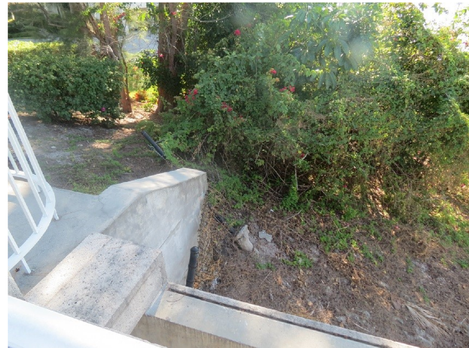
PHOTO 12 - REPLACE FENCE AT END RIGHT QUADRANT.
