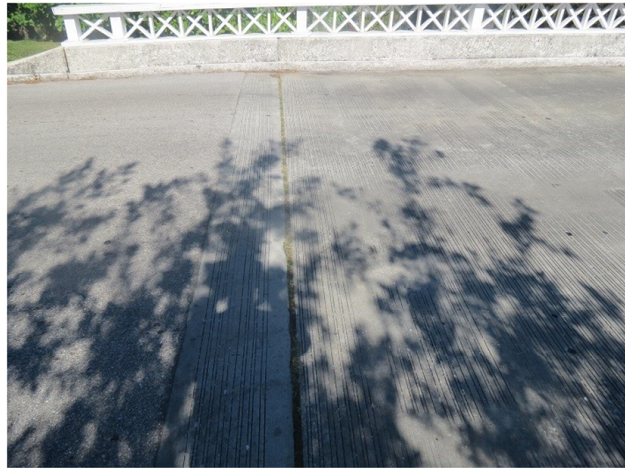
PHOTO 1 - EXPANSION JOINT AT END BENT 1
