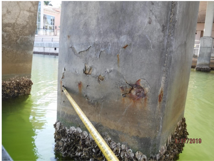
PHOTO 9 - DELAMINATION ON PILE JACKET 3-7.
