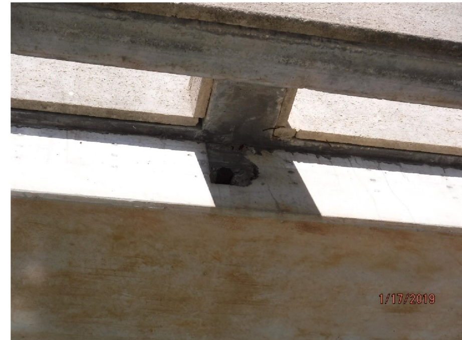
PHOTO 4 - PATCH POST-TENSION DUCT.
