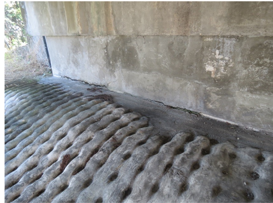
PHOTO 10 - UNDERMINING AT END BENT 5
