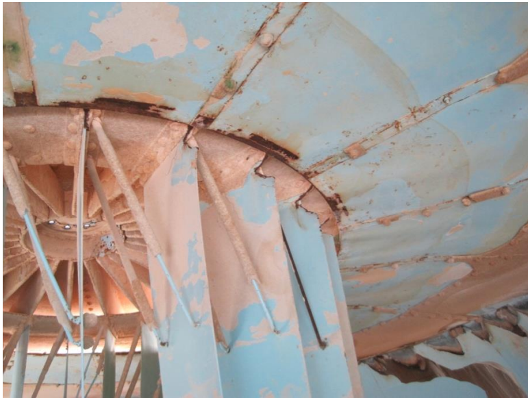
Underside of deck plate assembly with impellor/rotor assembly
