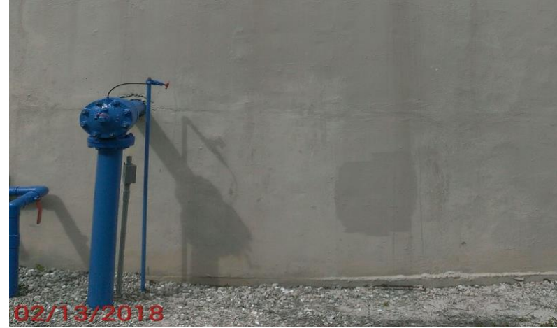
4" sludge flushing line on exterior of tank
