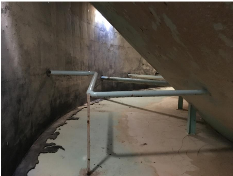
4" sludge flushing line in void area of tank
