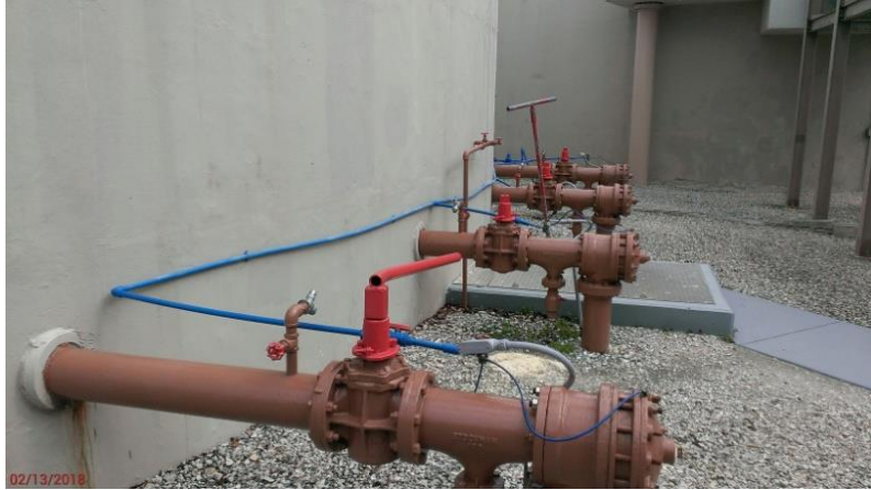
View of sludge blow off lines on exterior of tank
