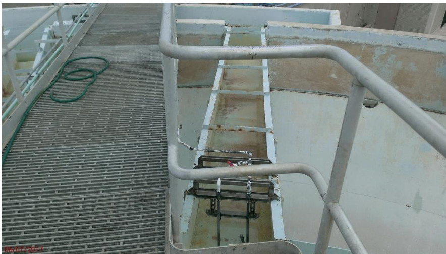
Catwalk with effluent launder; note chemical piping
