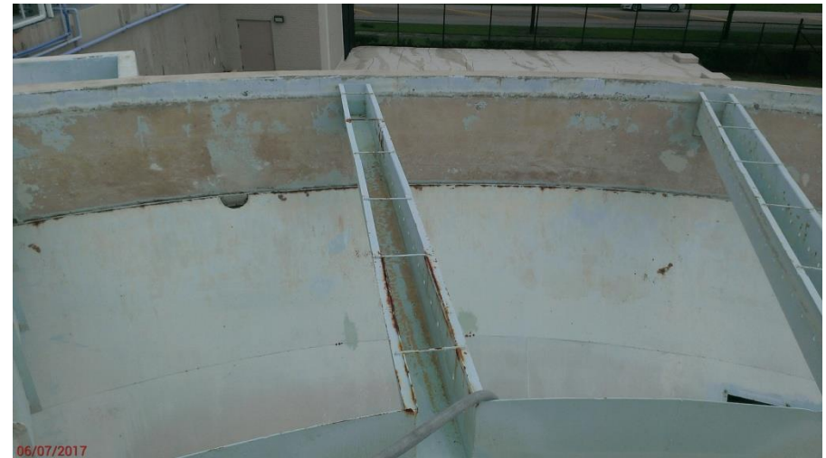
Radial launder, sloped steel plate with equalization opening
