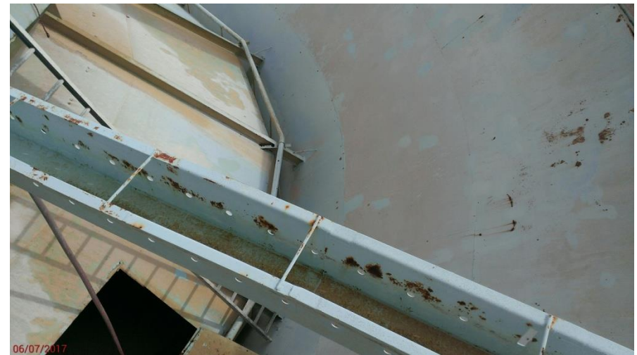
Looking down at hood and rafters; note sludge flushing piping
