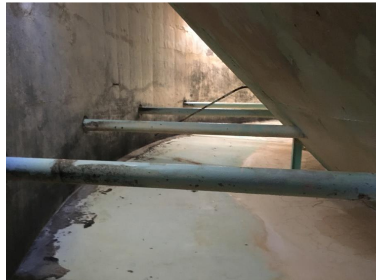
6" sludge blow off lines in void area of tank
