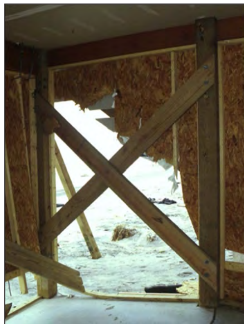
Figure 9: Cross bracing that interfered with the failure of a breakaway wall
