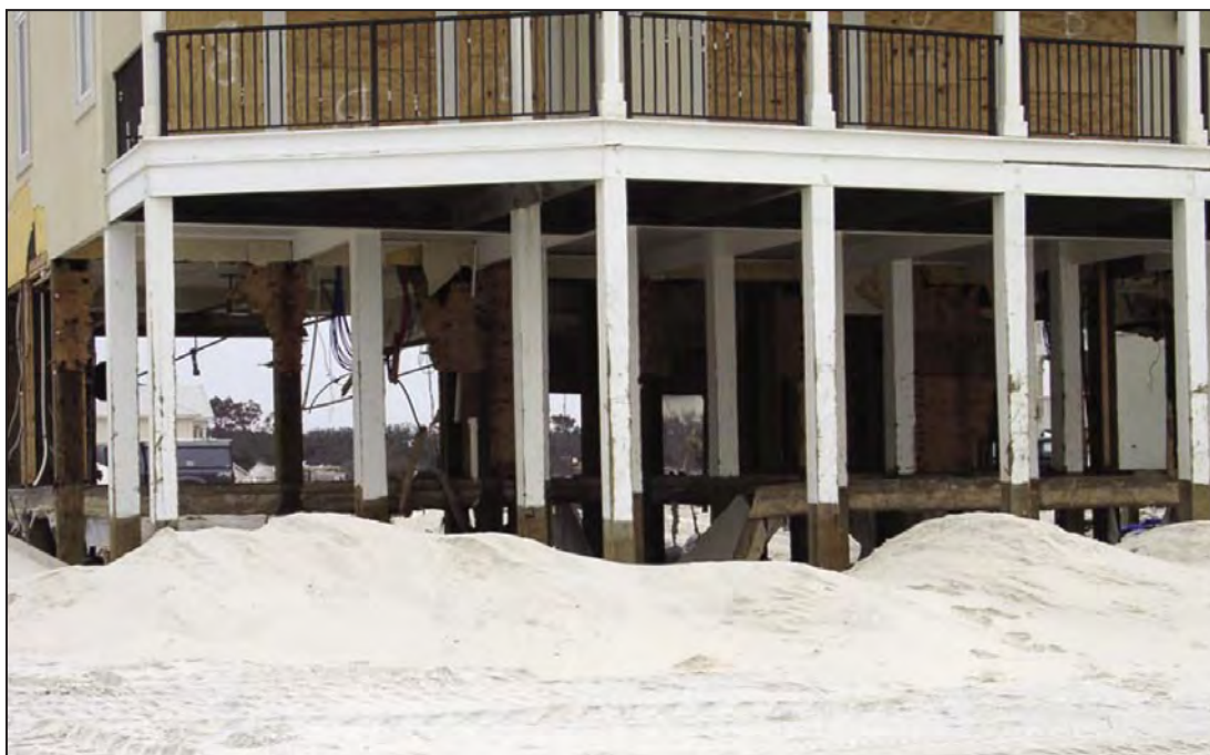
Figure 4: Breakaway walls under an elevated building that were removed by waves (i.e., performed as intended) during Hurricane Ivan in 2004 (Gulf Shores, AL)
