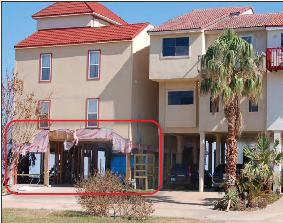
Figure 7: Non-compliant joint detailing, resulting in the propagation of damage above the lowest floor when the breakaway walls broke away during Hurricane Ike in 2008 (Seabrook, TX)
