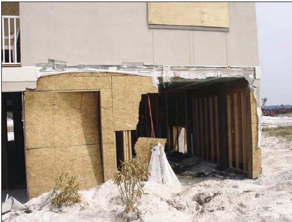
Figure 10: Non-compliant breakaway walls that were nailed over the piles and floor beam, preventing a clean break during Hurricane Ike in 2008 (Gulf Shores, AL)
