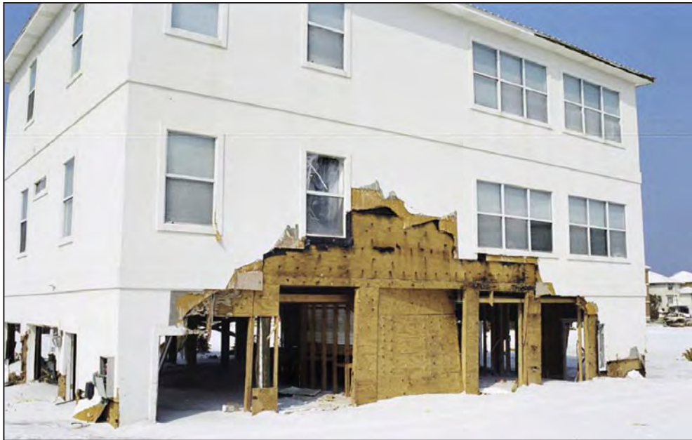
Figure 6: Damage caused by waves running up the exterior wall prior to dislodging of breakaway walls during Hurricane Ivan in 2004 (Pensacola Beach, FL)
