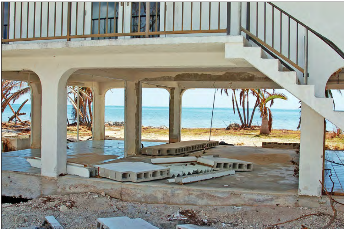
Figure 5: Unreinforced masonry breakaway walls removed by waves (i.e., performed as intended) during Hurricane Irma in 2017 (Monroe County, FL)
