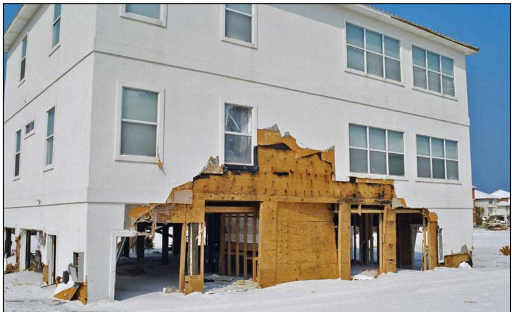
Figure 7: Breakaway wall that did not break away, which led to wave runoff and contributed to flood damage on the side of the elevated building
