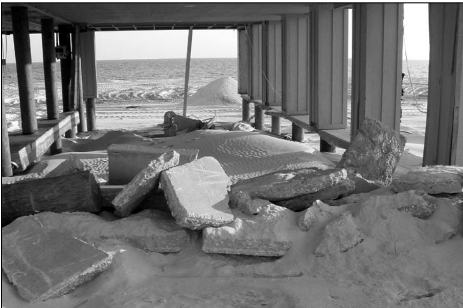
Figure 21: Unreinforced slab that broke apart without imposing loads on the foundation
