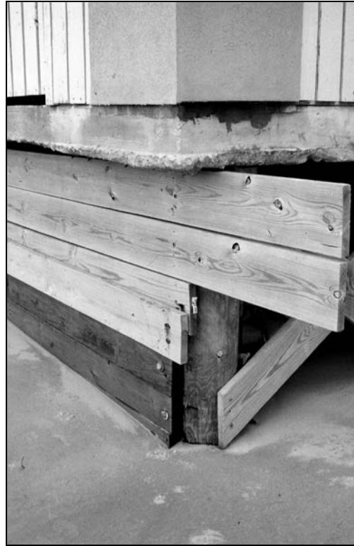
Figure 25: Shore-parallel timbers attached to a pile foundation that were intended to act as a bulkhead but constituted an obstruction and are not permitted
